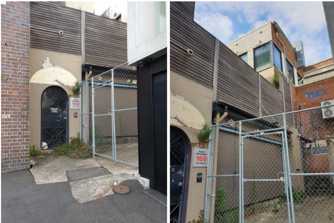
Figures 21 & 22: Rear of the former Golden Apple building at 169 Victoria St viewed from Hourigan Ln, facing east (left) and rear of the Piccadilly Hotel building at 171-173 Victoria St viewed from Hourigan Ln, facing south-east (right)
